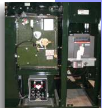
MiniSub with Primary Auto Transfer Switch
