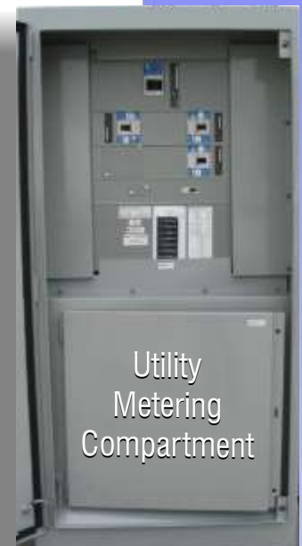
Side Distribution Panel with Utility Metering Compartment
