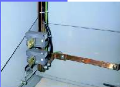
LV Grounding Connection
