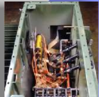
Bay-O-Net and backup current limiting fusing
