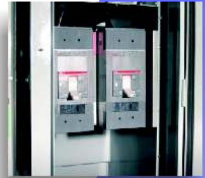
Low Voltage Breakers
