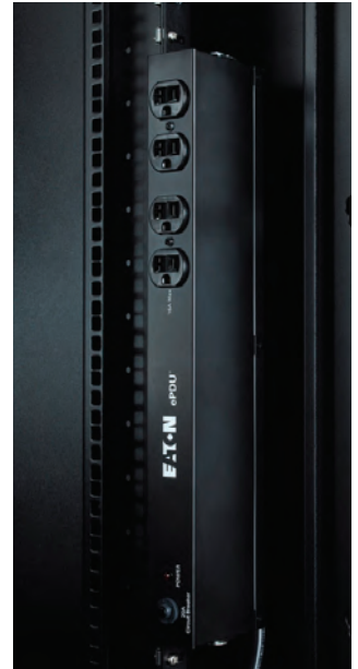
ePDU mounted vertically in rack
